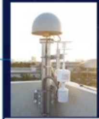
Quasi-Zenith Satellite System (QZSS)
